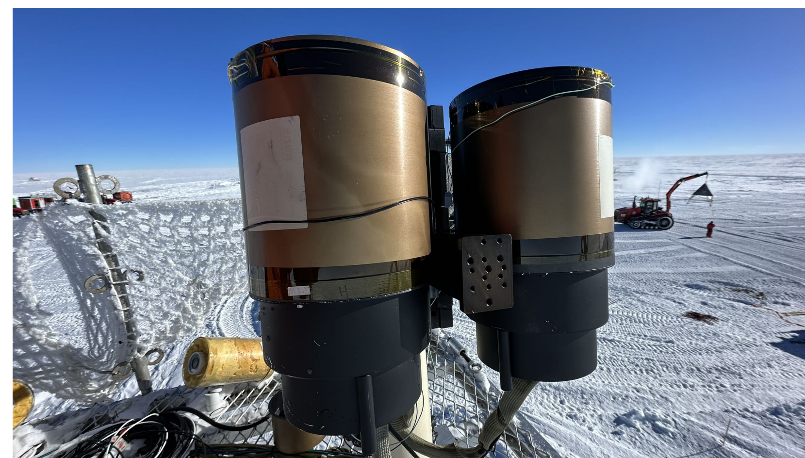
Figure 5: Installed in 8m tower in DomeA by China 39th, 40th Antarctic Expedition team.
